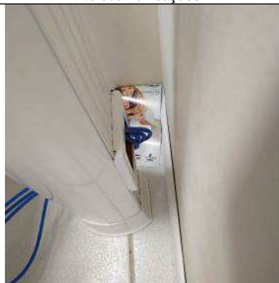
Figura 22E - Patch cords
