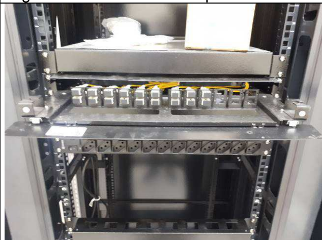
Figura 46E: rack 01 (principal)
