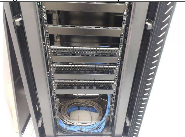
Figura 45E: rack 01 (principal)
