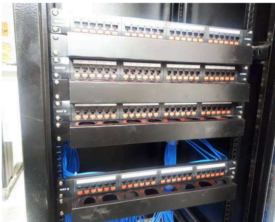
Figura 23E: Rack, patch pannel
