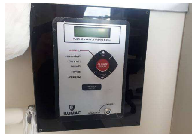
Figura 26E: Painel repetidor SDAI
