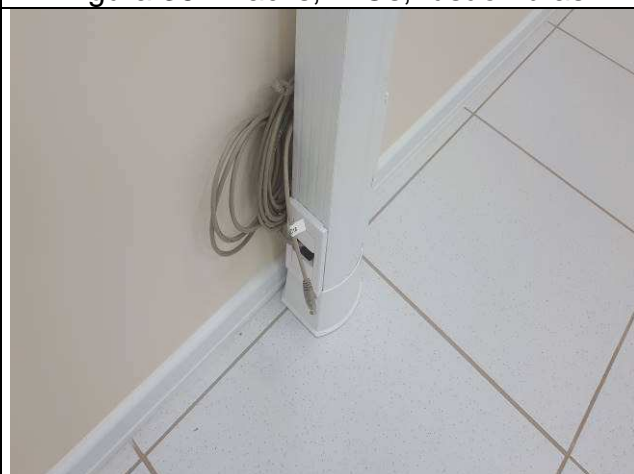
Figura 38E: patch cords 10m
