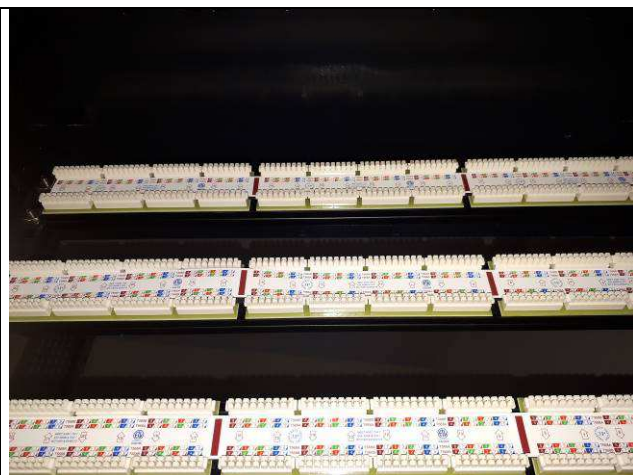
Figura 32E: rack principal
