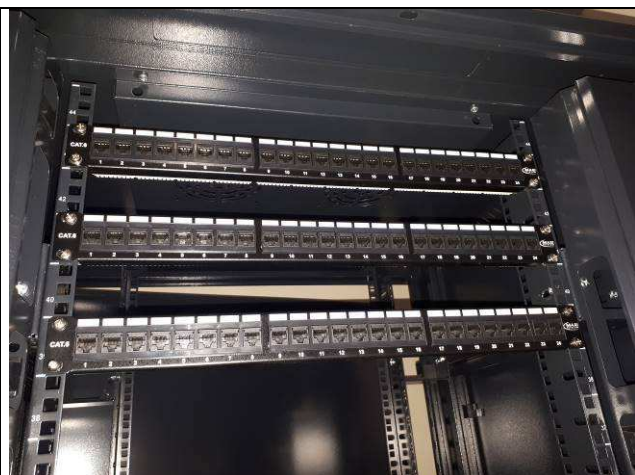
Figura 31E: rack principal
