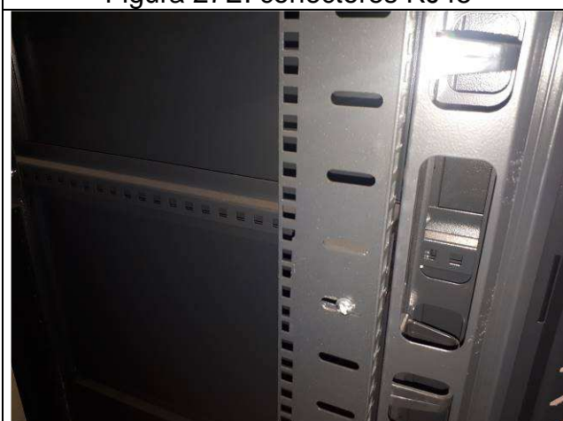
Figura 29E: rack principal
