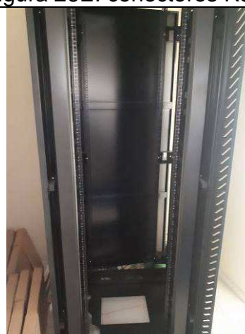
Figura 28E: rack principal
