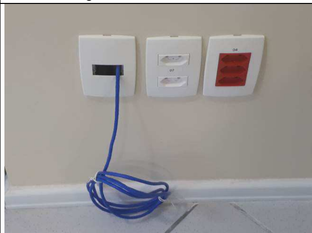
Figura 33E: patch cords
