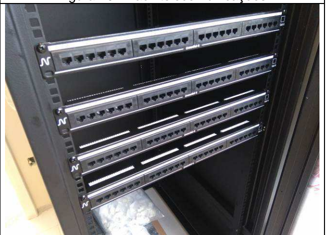
Figura 42E: rack - patch panel
