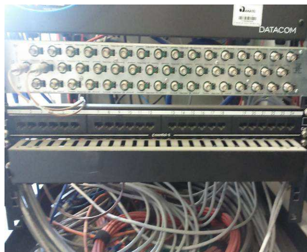
Figura 26E: Patch panel cat. 6
